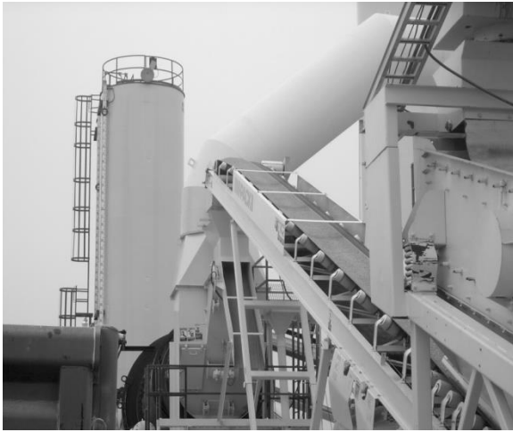
Dryer-drum Plant Cold Elevator Conveyor
