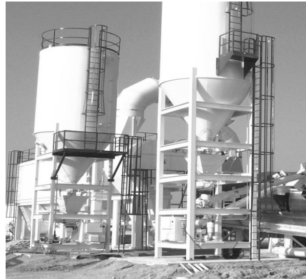
Dust storage tanks w/weigh pod
