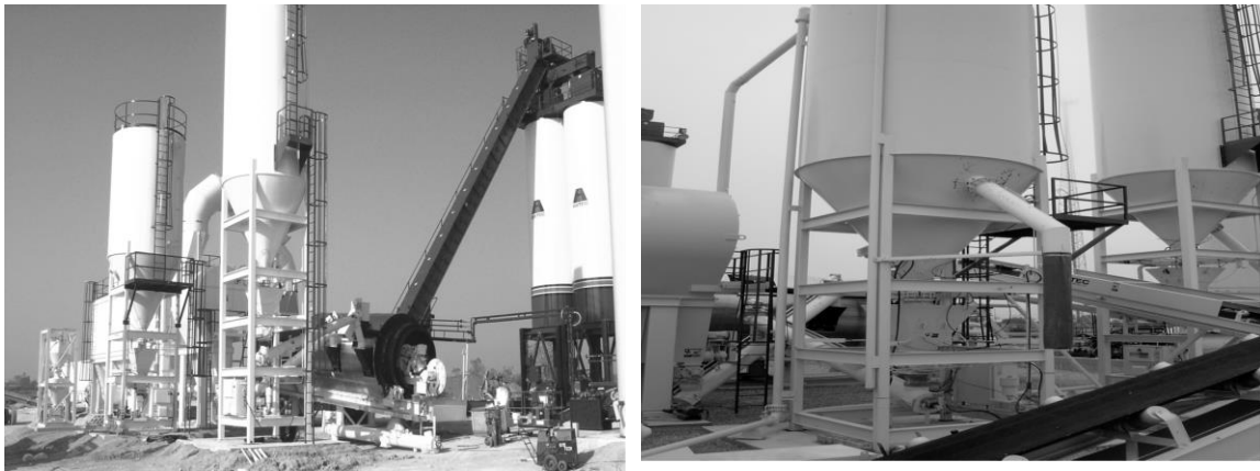
Mineral Filler Storage Systems
