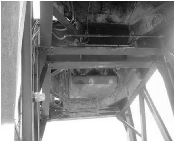
Silo Discharge Gate
