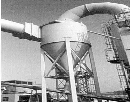
Cyclone Primary Dust Collector
