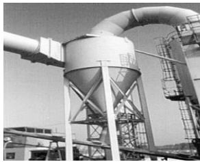
Horizontal Cyclone Collector
